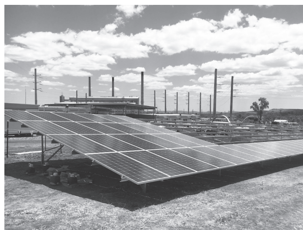
42.5-MW Collinsville Solar PV Project, Queensland, Australia
