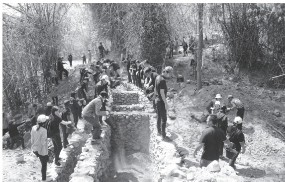
“Check Dam construction” volunteers’ activity at the community forest at Ban Phu Ron, Suphan Buri
